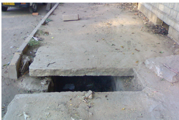
Missing links in infrastructure aiding pedestrian injury and death in Bangalore
